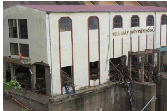
Figure 2. Damage of Ho Ho powerhouse caused by debris flow and driftwood.
